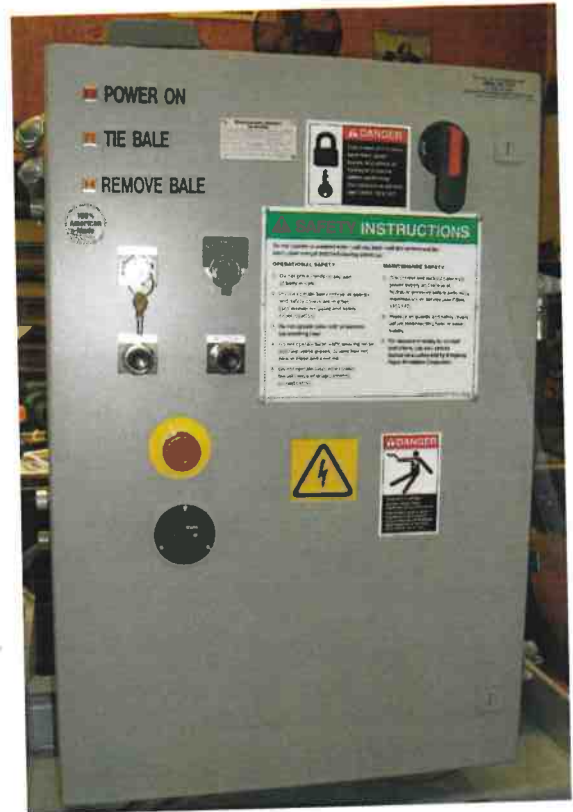
Baler Control Panel
